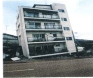
Fig. 5 Soft first storey collapsed, upper part of the building fall onto the ground, (kachchh, 2001)
