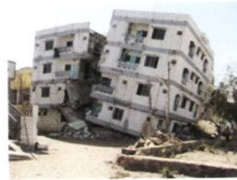
Fig. 6 Soft Storey (Open Plinth), Vertical Split between two blocks (Bhuj)
