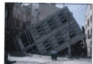
Fig. 3 The solid building tilted as a rigid body and the raft foundation rises above the ground
